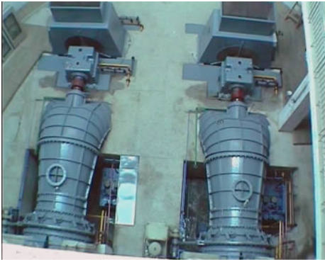
The hydroelectric generator set
