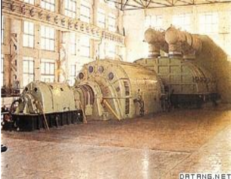
The steam turbine generator set
