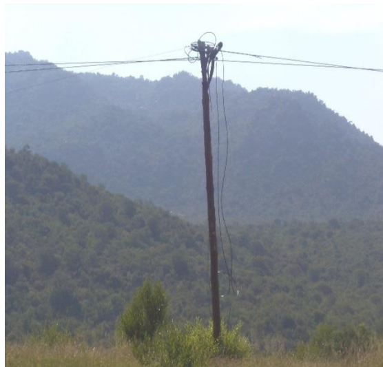
Figure 5.2: Vandalised telecommunication infrastructures between Jane Furse and in Ga-Malekane village.
