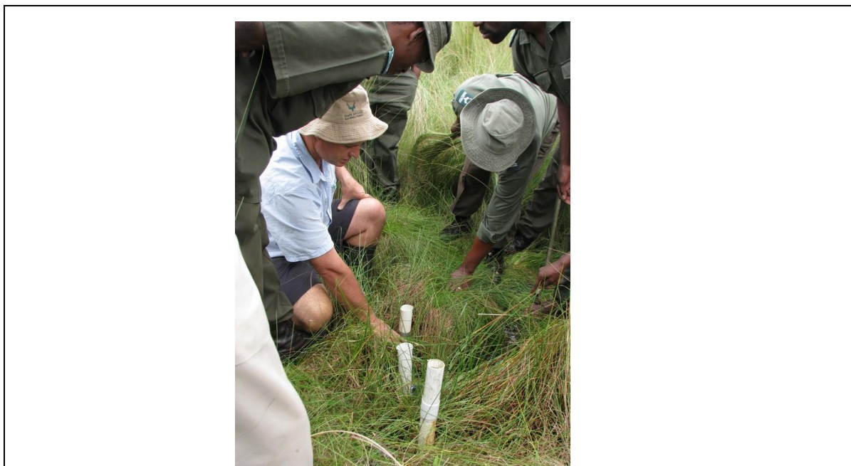
Figure 10. An example of a piezometer nest made up of three PVC pipes forming a well and two piezometers that extend to various depths of the substrate
