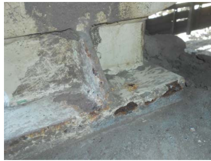
Figure 5. Corrosion damage evident only after debris has been removed.
