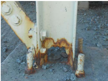
Figure 1. Localized corrosion that is causing the loss of load bearing capacity of a structural beam. How long will it last?
