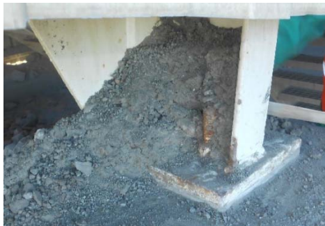
Figure 4. Debris obscuring the metal surface
