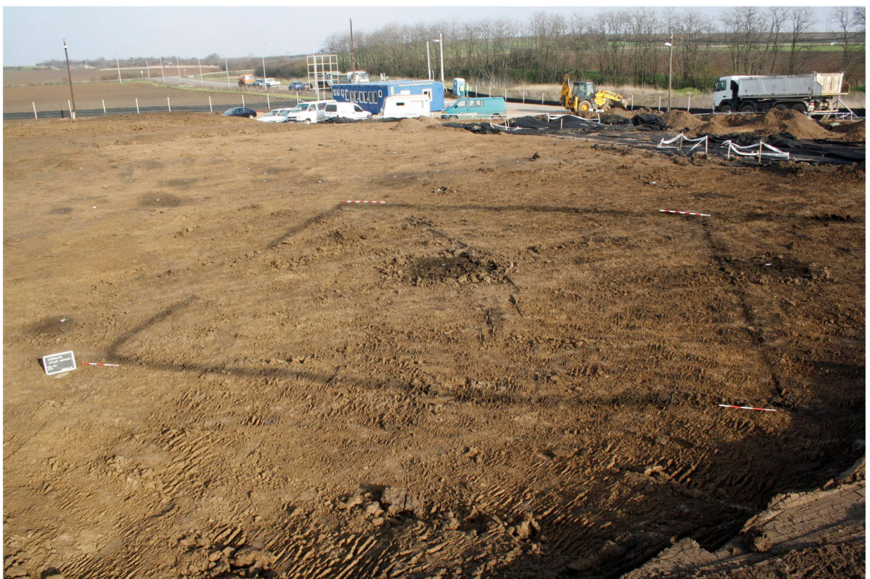
Fig. 2. Gyöngyös – Külső-Mérgecs-patak 1. Topsoil stripping on the site (above) and the ground surface of the Late Iron Age cemetery (below) (Photos: K. Tankó).
