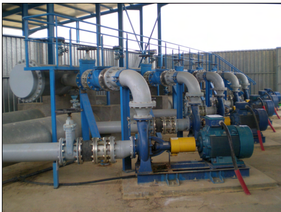
Fig. 35. Bombas sector XXI
