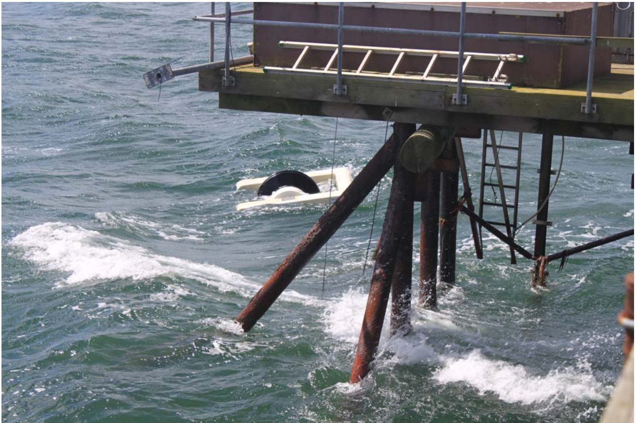
Figure 5. Pressure sensor is on the pole on the right side of the ladder.
