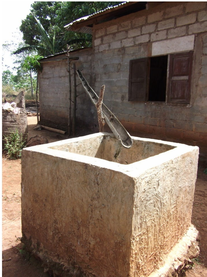
Photo 4.3 Rainwater collecting tank and bamboo pipe, Triloka area
