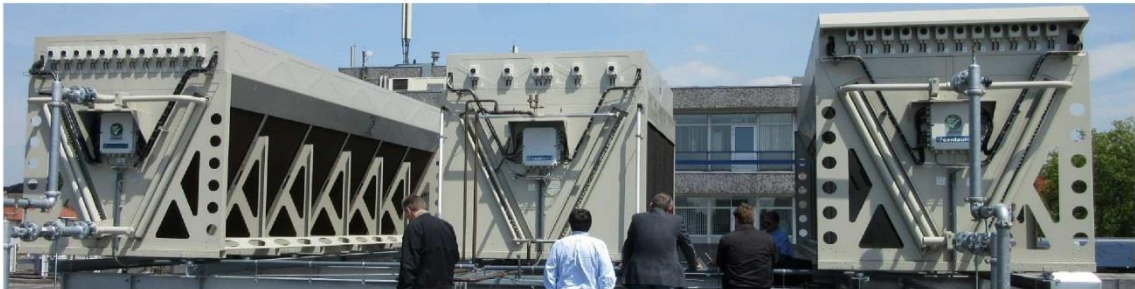
1x gas cooler transcritical (390kW) e 2x arrefecedores secos (2x 200kW) fornecidos e comissionados para a loja bandeira da Royal Ahold em Eindhoven 1x transcritical gas cooler (390kW) and 2x dry coolers (2x 200kW) supplied and commissioned for the flagship shop of Royal Ahold in Eindhoven
