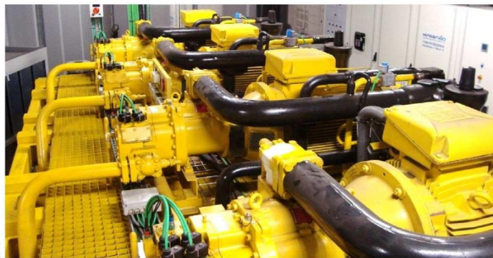
Chiller de compressores de parafuso Screw compressor chiller rack
