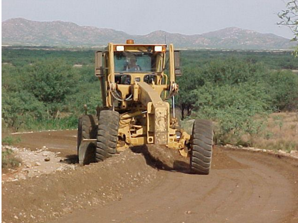
Figure 1-3: Machinery blending soil with stabilizer product in Buenos Aires NWR [Surdahl et al, 2005].
