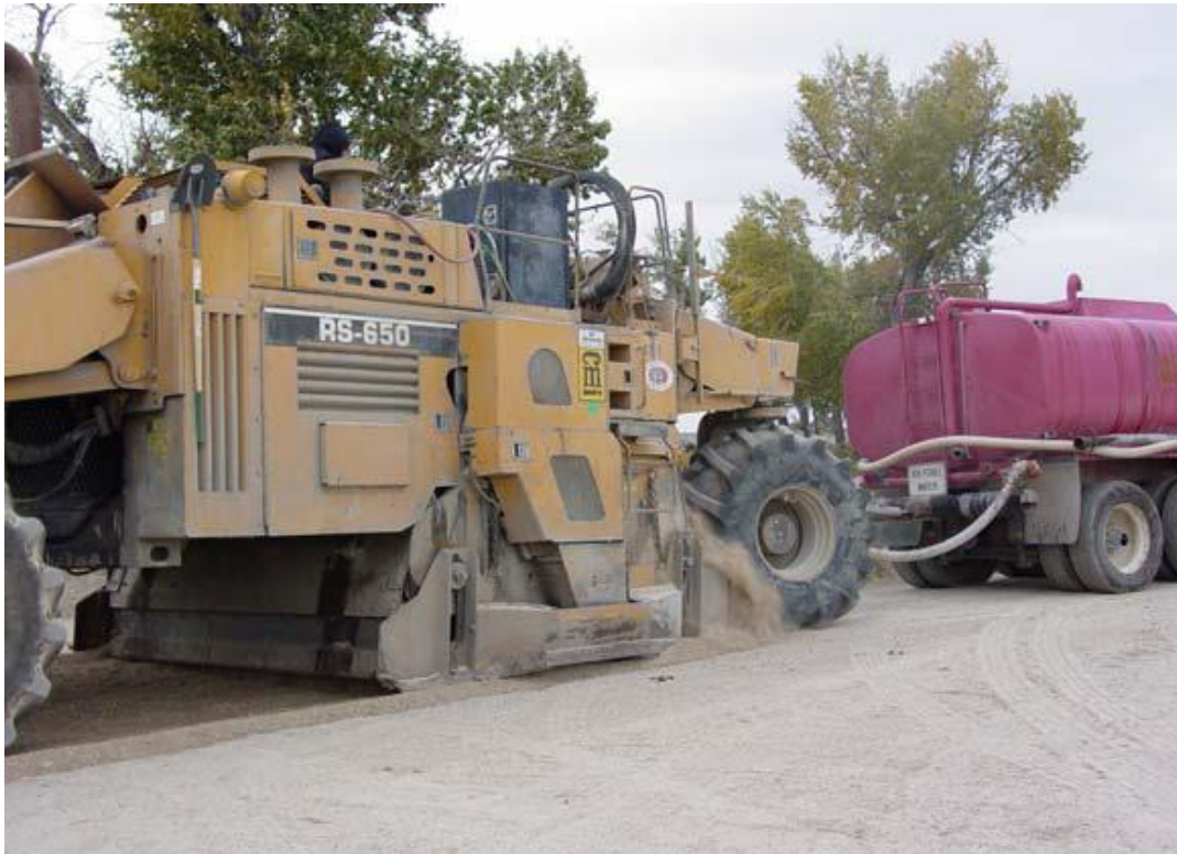
Figure 1-5: CMI Pulverizer used to compact and grade soil in Seedskadee NWR [Woll et al, 2008].
