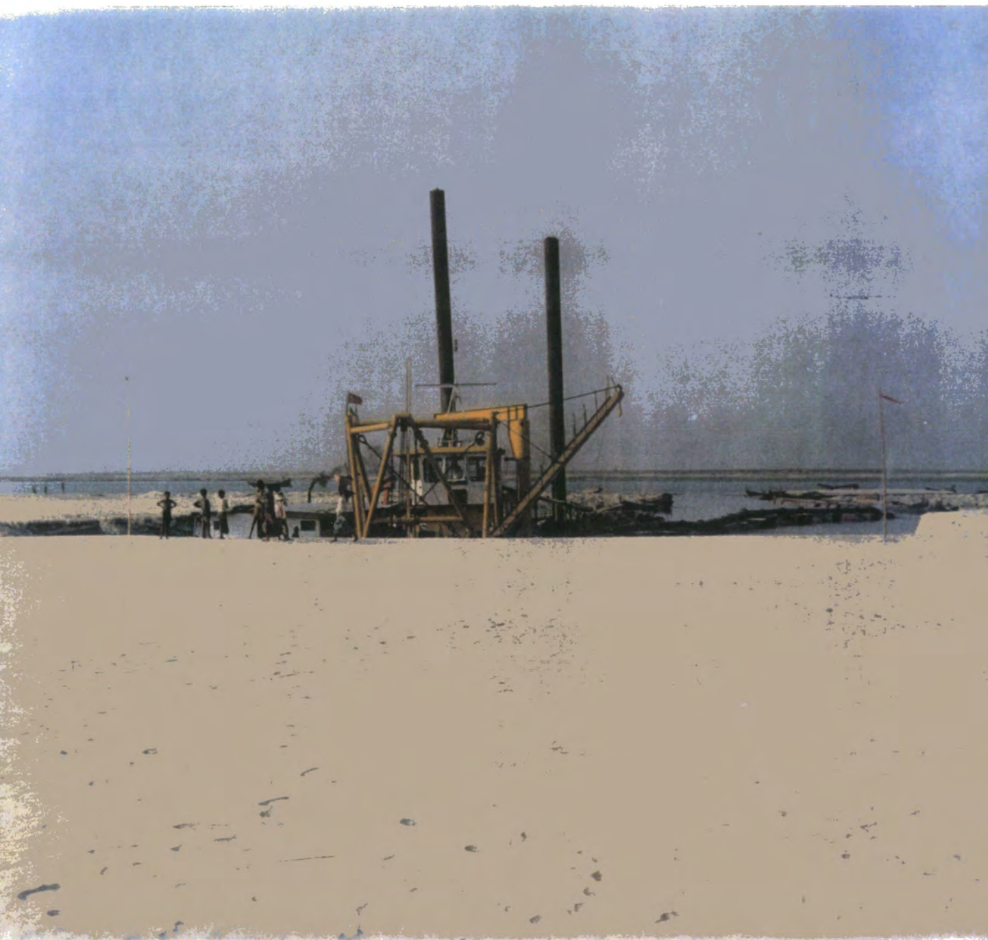
Photograph 4 Unsuccessful effort to make the Gorai's mouth navigable Source: B.W.D.B., March 1993
