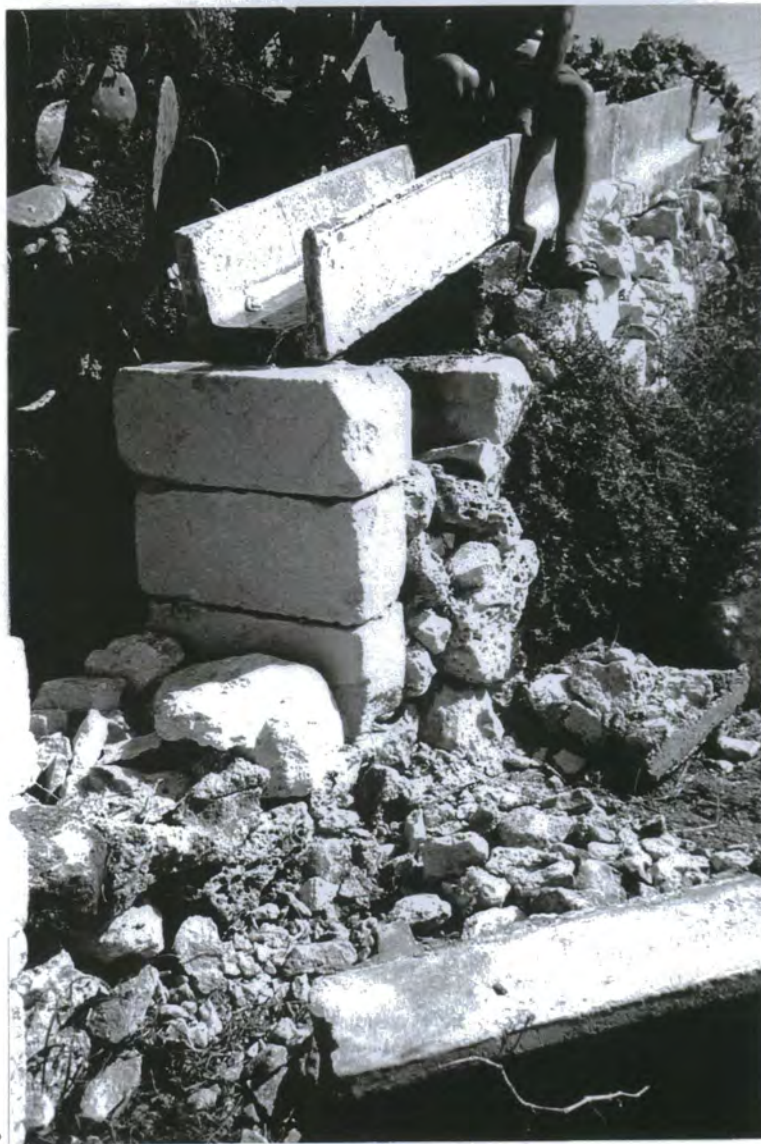
Plate 5.10. Water is still flowing in this collapsed channel, making repairs difficult.
