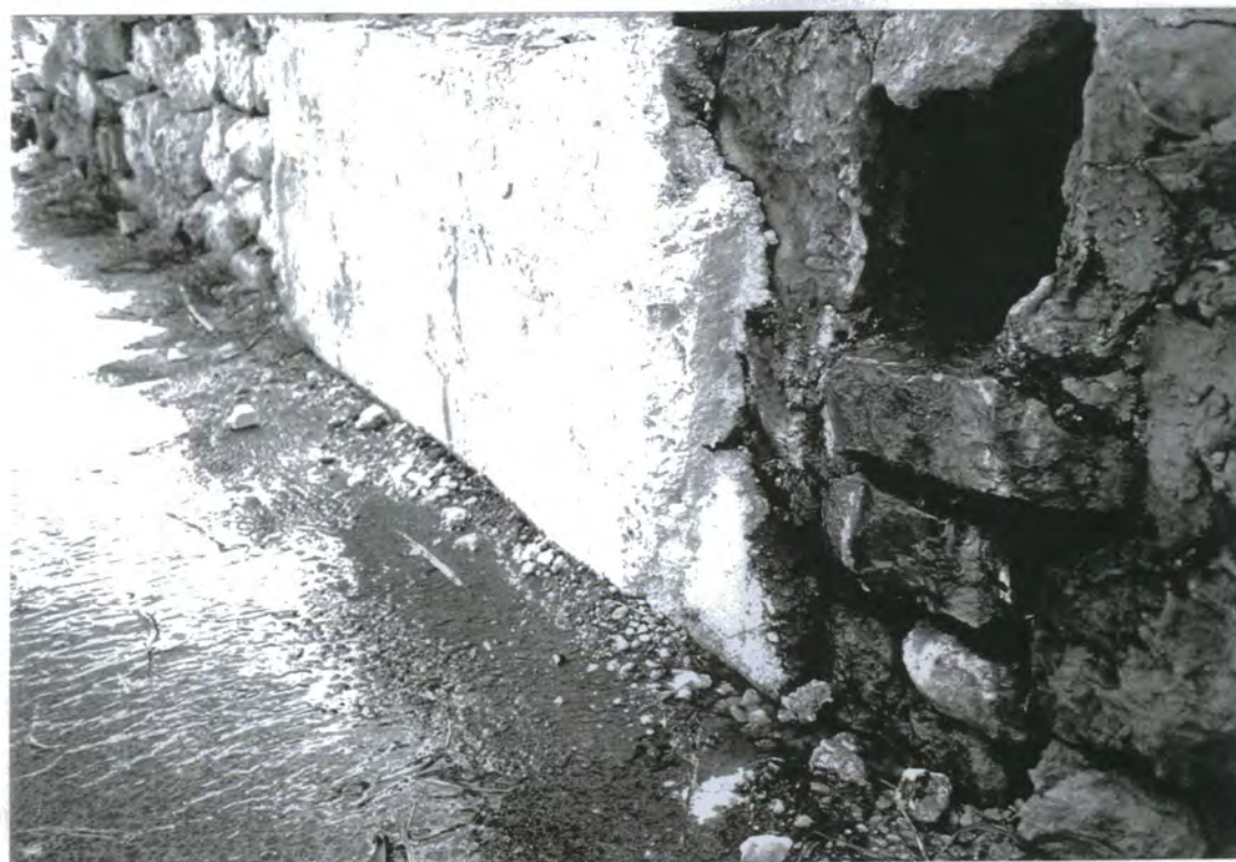
Plate 5.6. Large volumes of water leaking from a water channel. It can take several days before it is reported and repaired.
