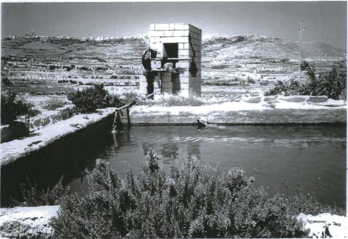
Plate 3.17. A diesel pump extracting groundwater in Gozo.
