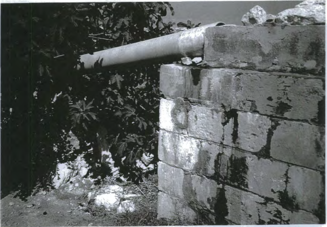
Plate 5.7. A low level leak in a water channel.
