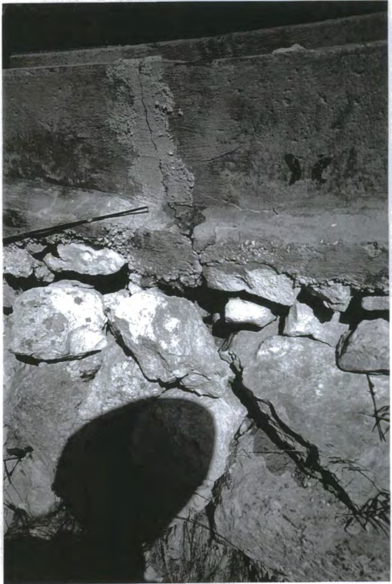
Plate 5.8. A small leak which is difficult to detect and represents a large water loss.
