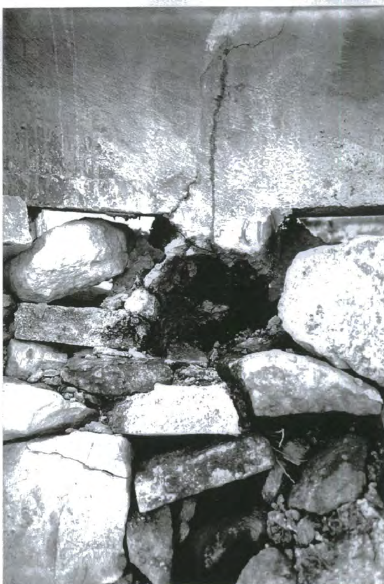
Plate 5.5. Water leaking from a crack in the water channel.
