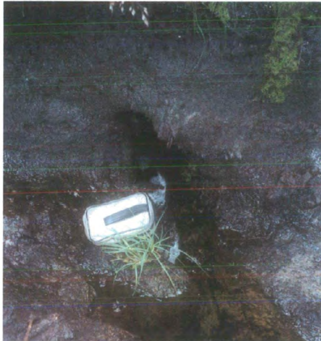
Figure 8.11. Seepage zone and pipe 8. a) Aspect of the valley, b) sinkhole with c) pipe
