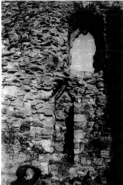
Plate 9 A Triangular Headed Mural Passage in the East Curtain Wall of Richmond Castle
