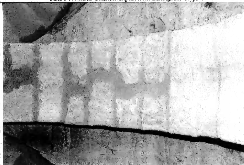
Plate 4 The Soffit of a Transverse Arch in the Crypt at Lastingham Church
