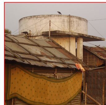
Figure 6.6: Overhead water storage tank in BT
