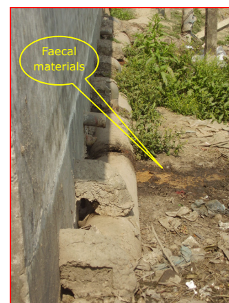
Figure 6.2: Photograph showing a broken pipeline of STL and exposed faecal material in MCC
