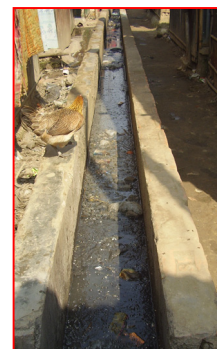
Figure 6.3: Condition of drains in BT
