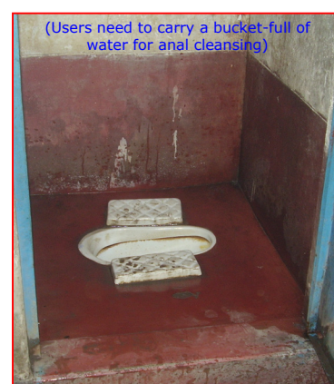
Figure 5.3: Absence of water source inside the latrine
