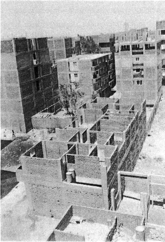
(47) Reinforced concrete frame & brick infill becomes a "traditional" way of building in informal settlements.
