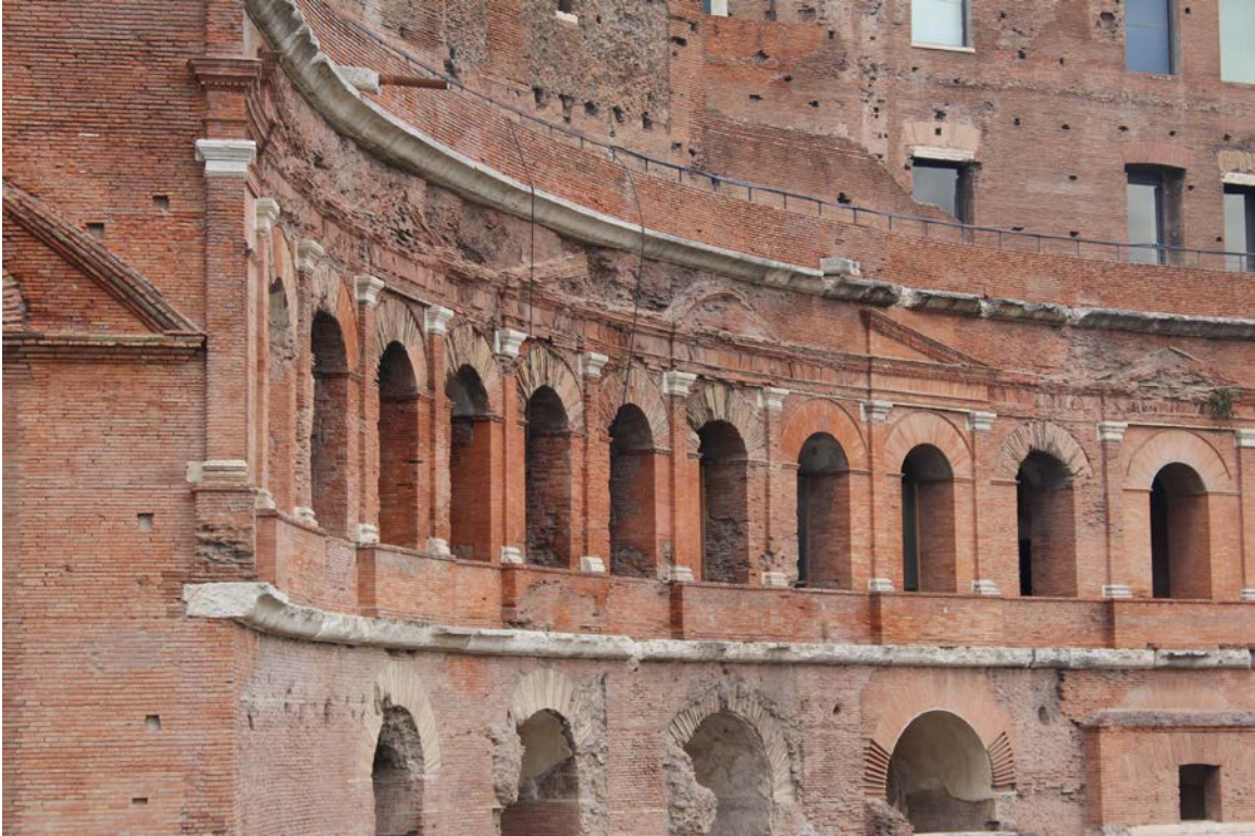
FIG. 114 Detail of the remains of Trajan's market: the whole complex is built of brick-faced concrete with travertine details. Similarly to Ostia, this new and simple use of the bricks, together with a façade system based on the rhythm of windows, determines the general appearance of Rome after the fire of 64.
