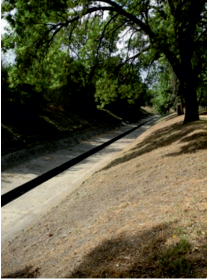
Photo 1. Straight canal of the Jasień river in the younger part of the city
