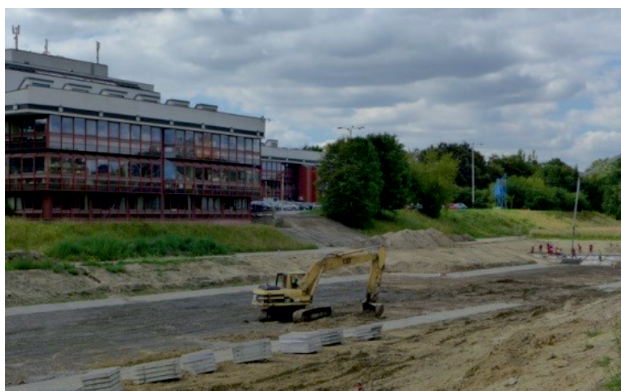
Photo 4. Reservoir within the floor of the Łódka river valley serves retentive and landscape functions
