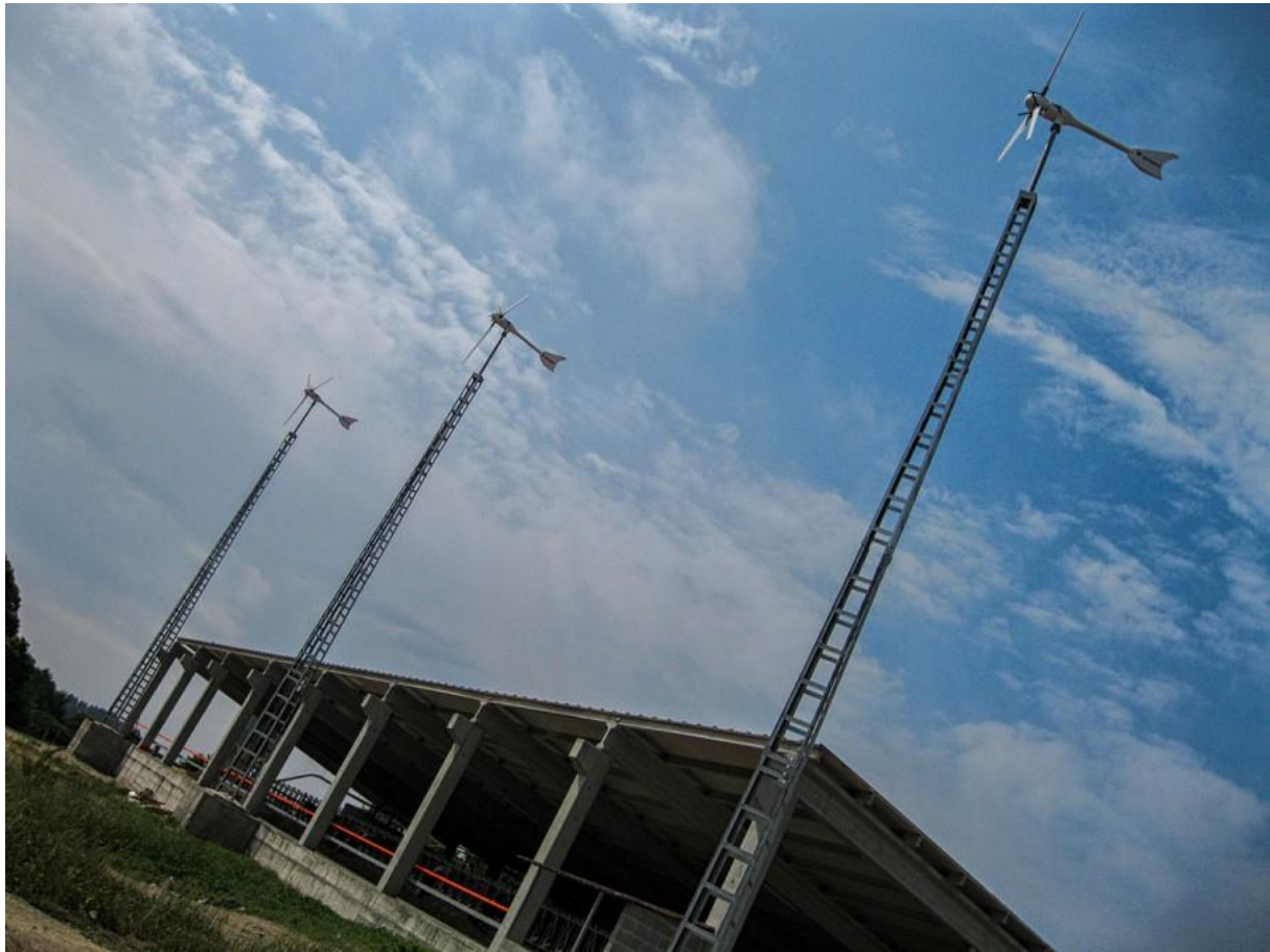
Figure 10. Image of the wind generators installed
