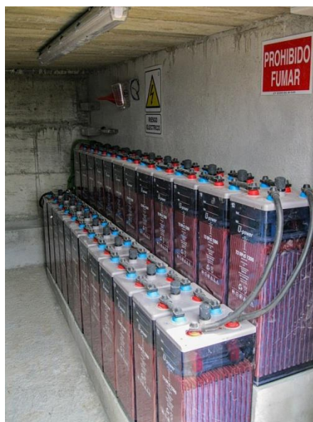
Figure 8. Installed battery bank
