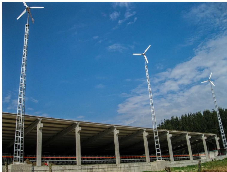
Figure 7. Installed wind turbines
