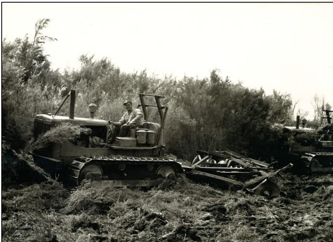
Figure 5: Crushing scrub on the Waihaha Development Block in 1956 (Source: Landcorp Farming Limited. Reproduced with permission)
