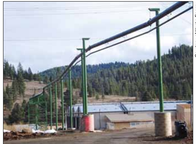
Figure 5-5—Steam line joining cogeneration boiler and kiln plant.
