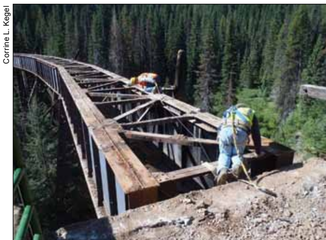
Figure 7-14—Dick Anderson Construction Company takes extra safety precautions while working on trestle repair.
