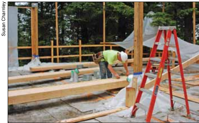
Figure 4-17—Employee of Ausland Builders working on the Redwood Sciences Laboratory second-floor addition.
