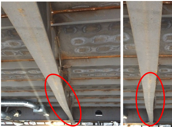
Figure 57: Production phase: defects in T-beams.
