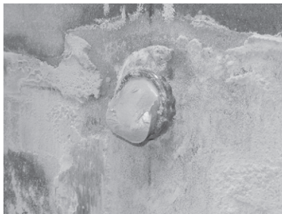
(a) Failed shear stud welded directly to the beam.
