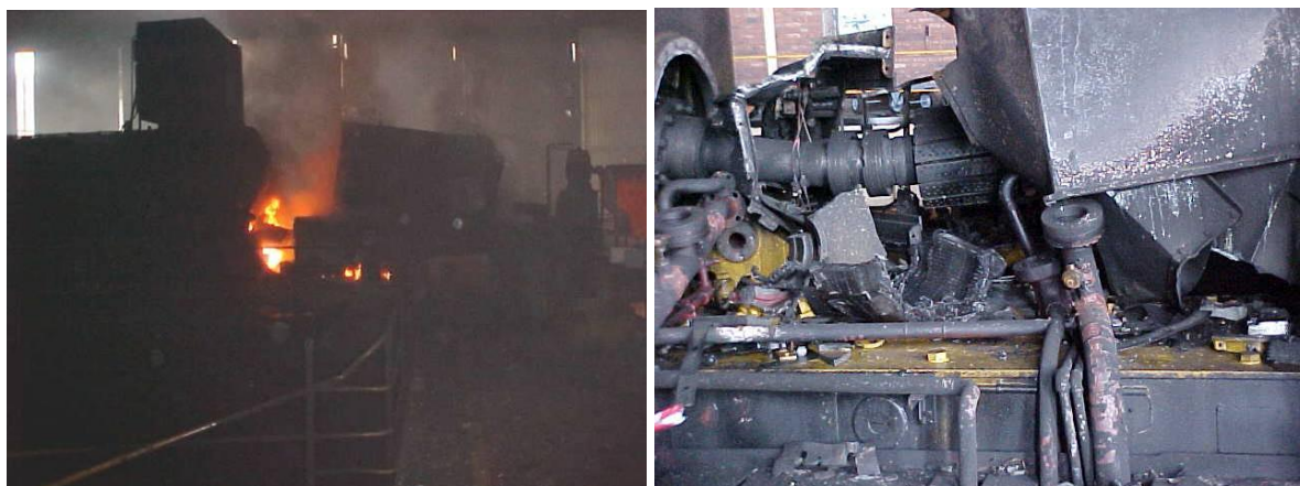
Figure 2-5 Catastrophic failure of LP rotor last stage blade
