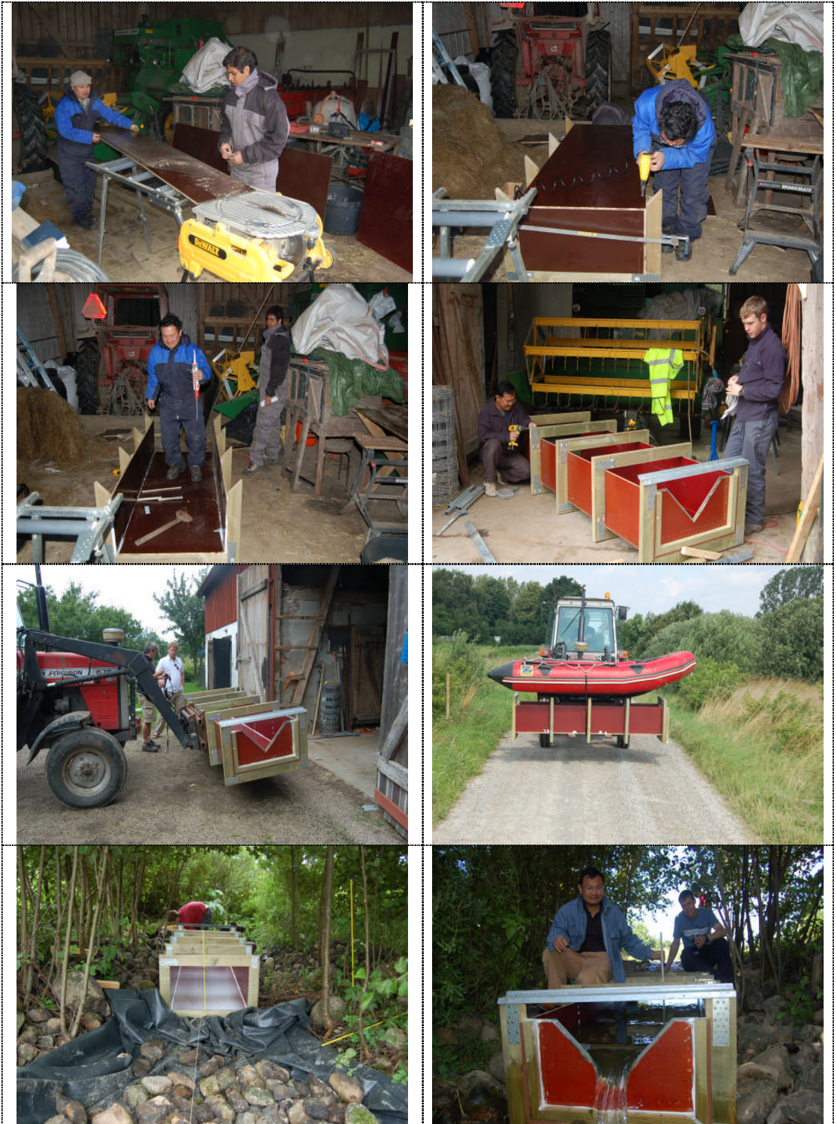
Figure 10-11. Pictures of design and build V-notch weir flumes for Lyby Field Pond.
