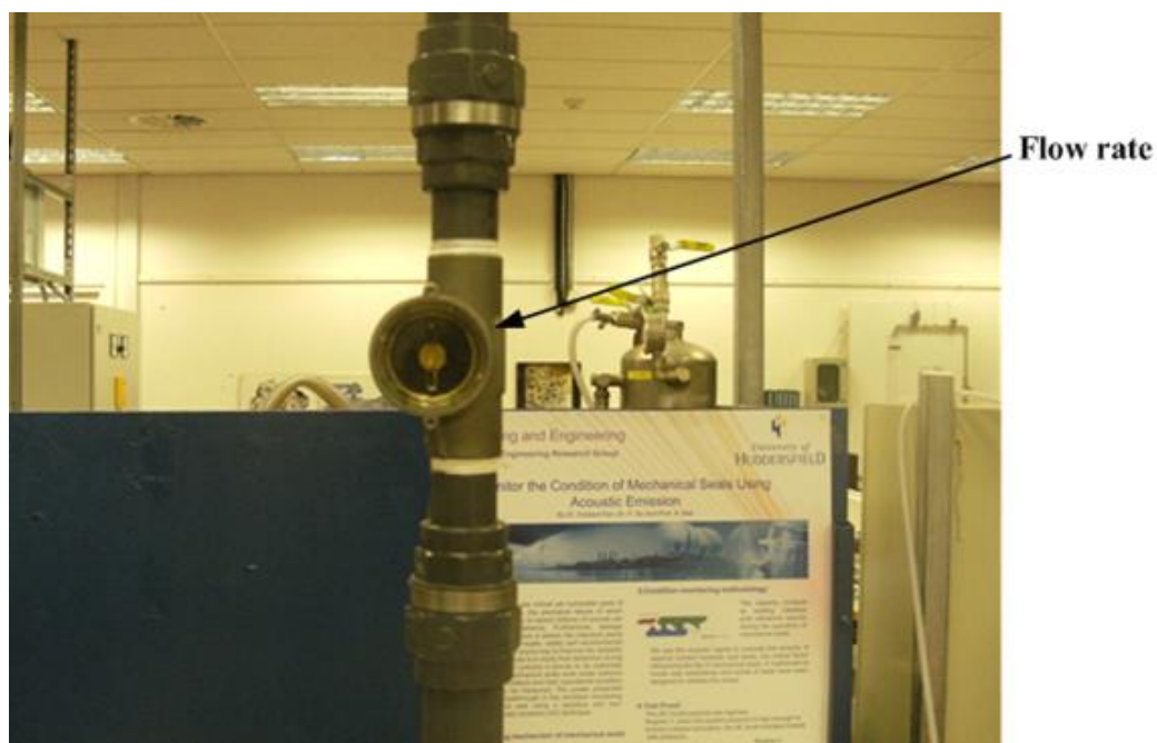
Figure 4-6 Gems water flow meter in flow line (refer to Figure 4-4)
