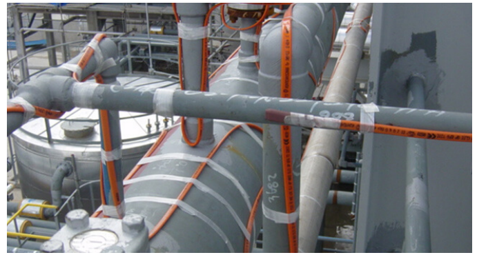
Fig. 4. Industry example of heat tracing placed on pipes [10].
