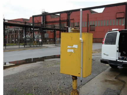
f) Other roadside electrical equipment.
