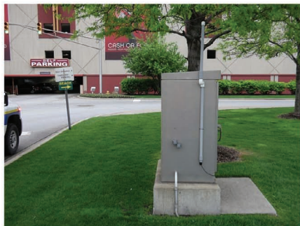
e) Traffic signal cabinet.
