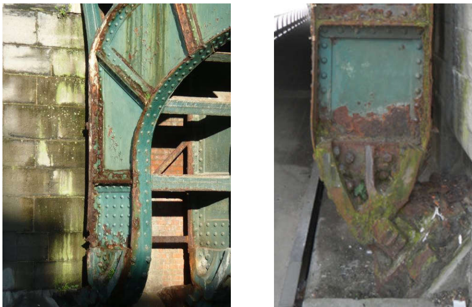
Fig. 2. Left : reduction of flange section Right : Corrosion of hinges
