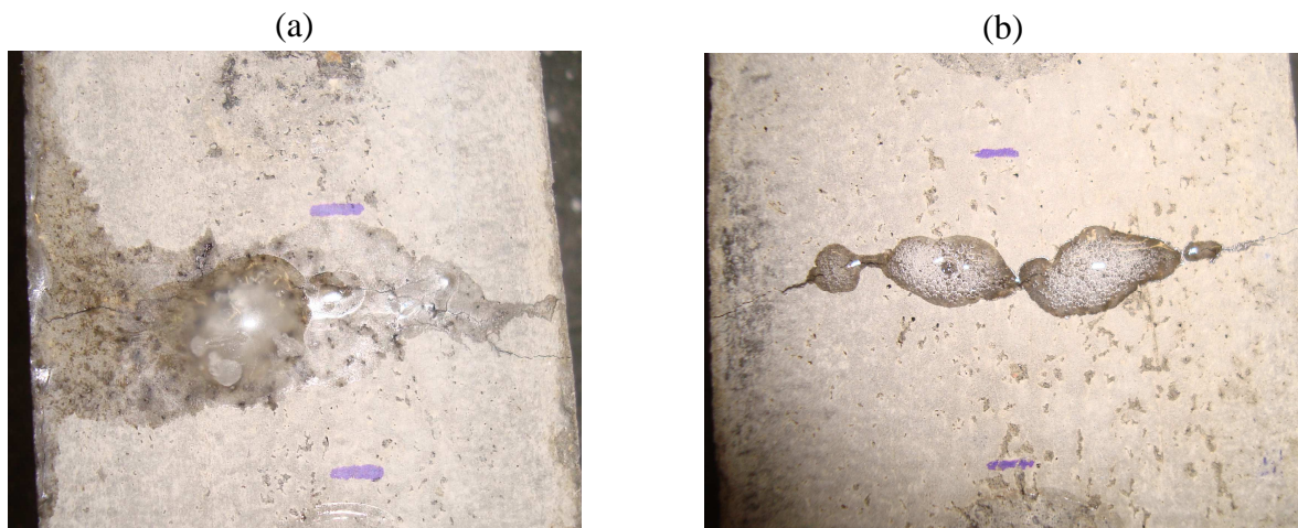
Figure 3: An example of (a) a specimen where a crack is healed by PU_LV and (b) a specimen where a crack is healed by PU_HV.
