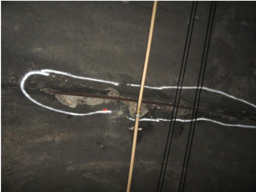
Fig. 42. Typical spalling and corrosion
