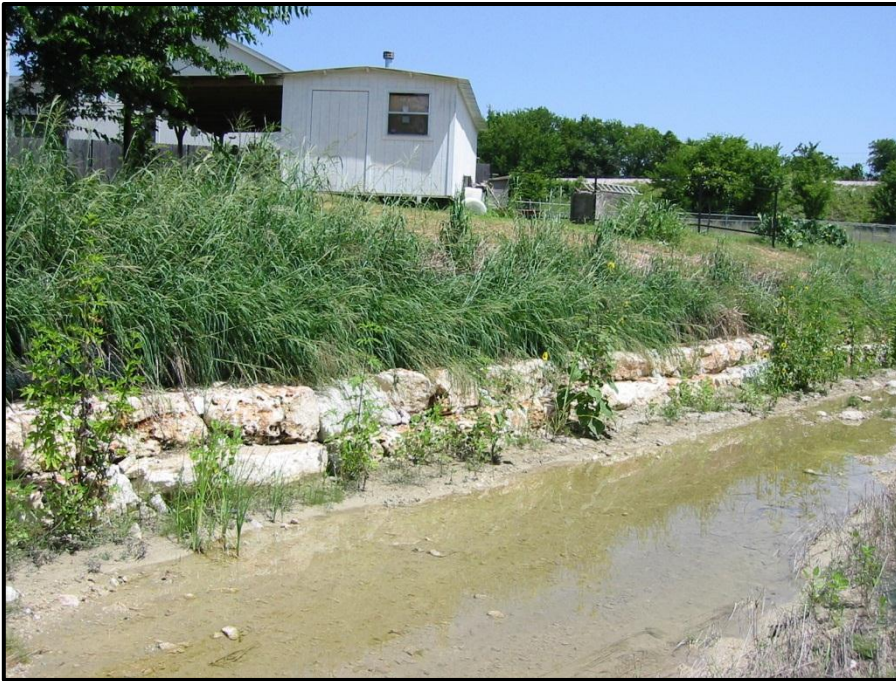
Figure A-11. Walnut Creek at Ritchie Drive after restoration in July 2004 (City of Austin 2004).
