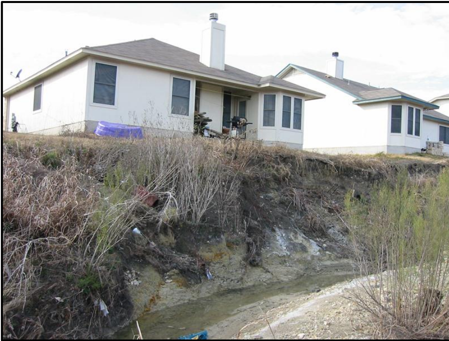
Figure 4. Houses adjacent to the eroded bank before restoration in 2003 (City of Austin).
