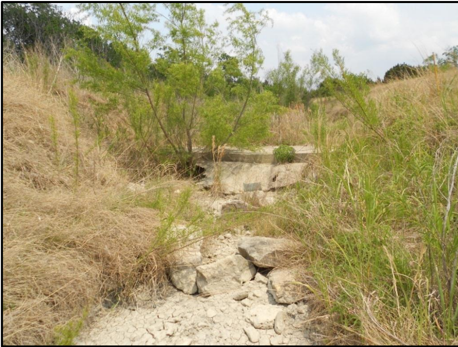
Figure 8. Front view of limestone rock riffle covered the petroleum pipeline, after restoration, 2011.
