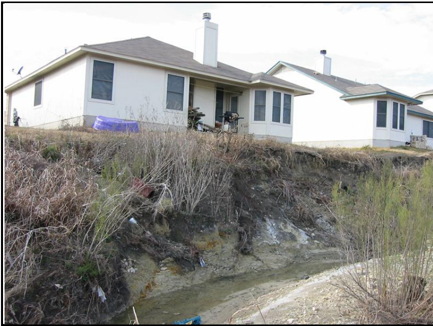
Figure A-1. Walnut Creek at 7315 Ritchie Drive before restoration in February 2003 (City of Austin, 2003).
