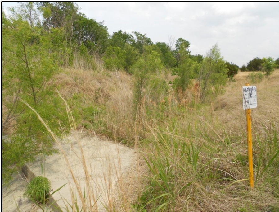
Figure 9. Side view of limestone rock riffle covered the petroleum pipeline, after restoration, 2011.
