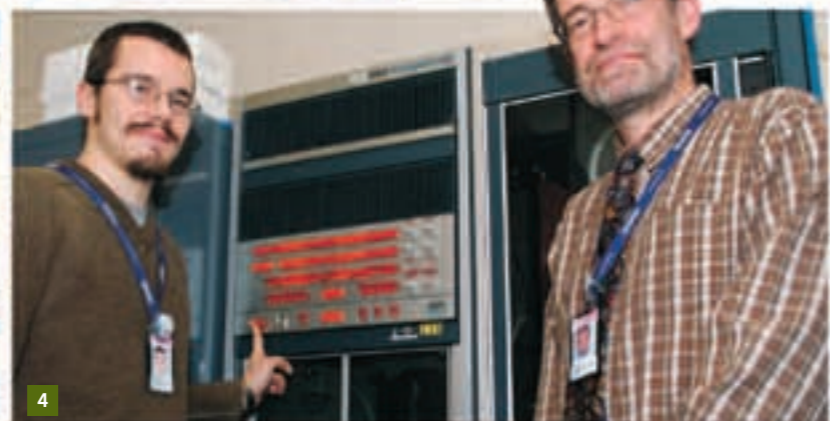
4. The last, original, operational GEC4000 series computer in the world is finally turned off after 28 years of service running ISIS controls by electronic engineer Steven Lochhead (who wasn't born when it was installed), watched by Controls group Leader Bob Mannix (who was, unfortunately!). 07EC1284
