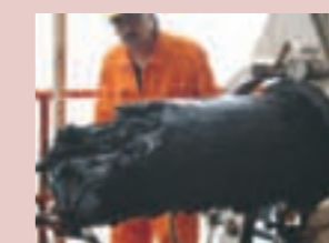
Photograph showing a crude oil pipeline blocked by asphaltenes and waxes.
