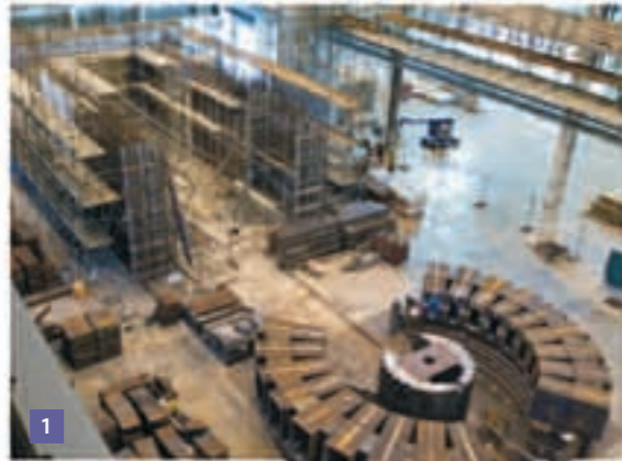
1. September 2006: First stages of the target station build. Rectangular viewports have been installed to allow neutron beams to travel out to instrument positions. 06EC3076
