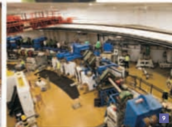
9. Installation of the TS-2 proton beamline extraction components in the ISIS synchrotron. 07EC3307
