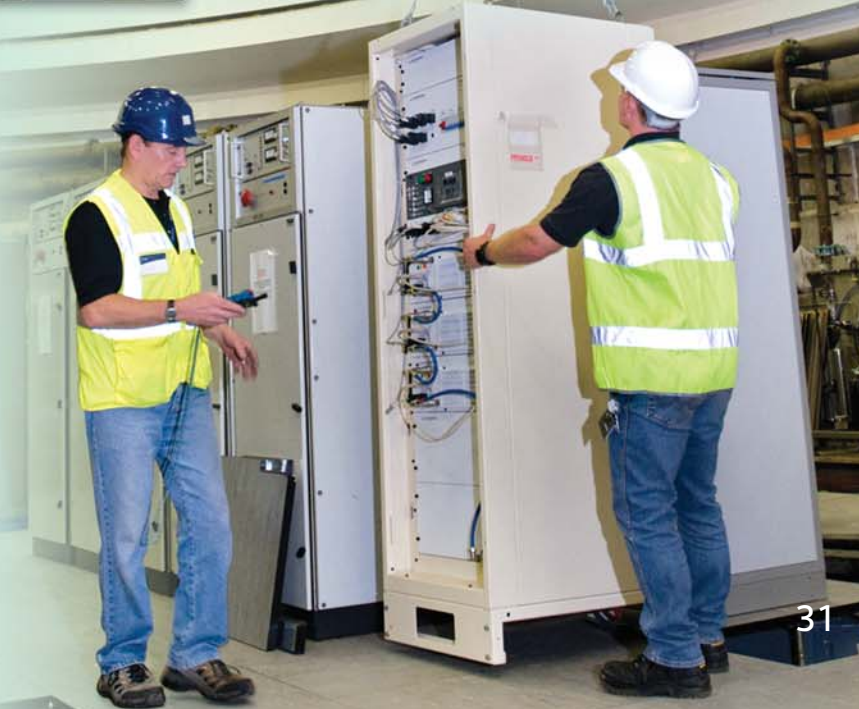
Right: Installation of new synchrotron steering magnet and trim quadrupole power supplies in the ISIS inner synchrotron. The new power supplies are capable of delivering a higher current output and a programmed current waveform with a slew rate of 300,000 Amps per second, twice that of the existing units.
