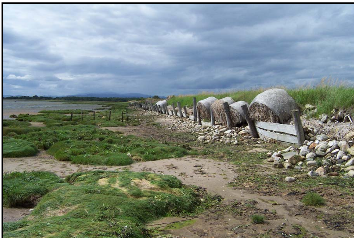
Figure 2.3: The eroding southern embankment prior to breaching. RSPB.
