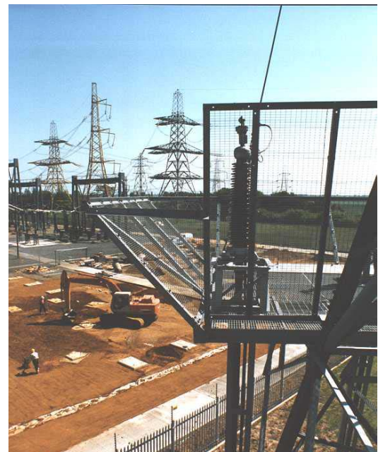
Plate 8.3 Cable Sealing Ends at Tower connected to overhead line
