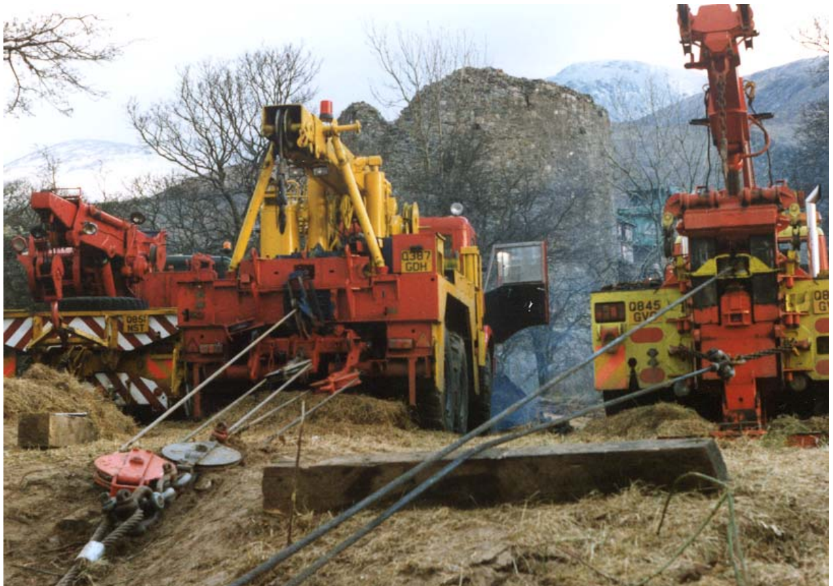
Plate 7.7 Three of the four mobile cranes used to pull the excavator out
