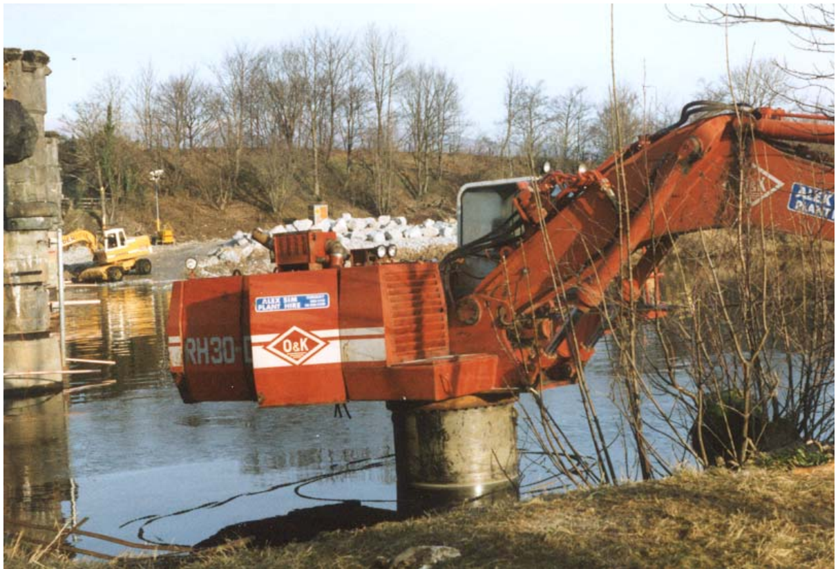
Plate 7.8 Excavator out awaiting repair (Note pieces of 'rock armour' visible in the background on the far bank)
