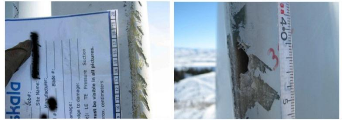
Figure 3. SLIGHT LEADING EDGE EROSION AND POTENTIAL THROUGH LAMINATE DAMAGE CAUSED, SOURCE: [8]
