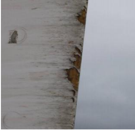
Figure 1. LEADING EDGE EROSION (presented without scale), SOURCE: [6]
