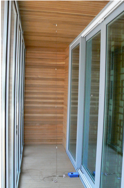
Figure 5 Column of air sensors
