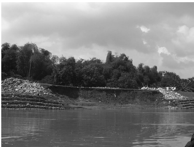
Figure 3. Global failure of gabion-reinforced section of embankment, which occurred during the first wet season after construction
