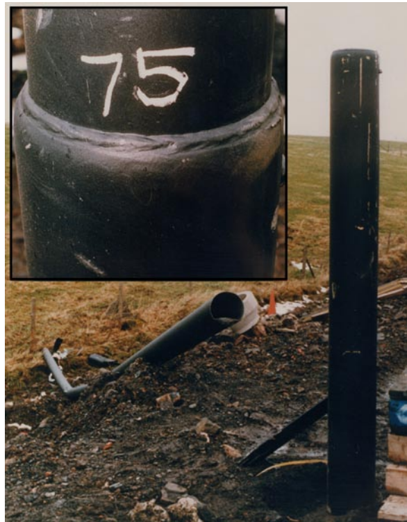
Figure 1: Low-cycle fatigue failure of 18m lighting column.
