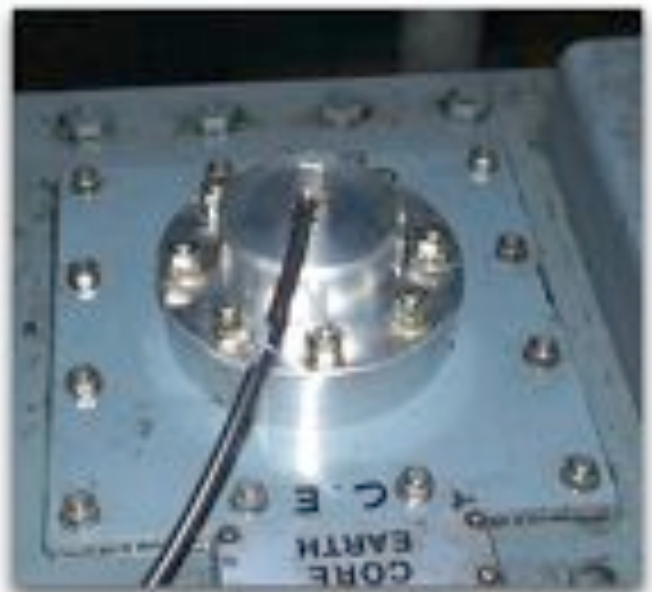
Figure 2. Externally mounted RF sensor on a power transformer inspection hatch.
