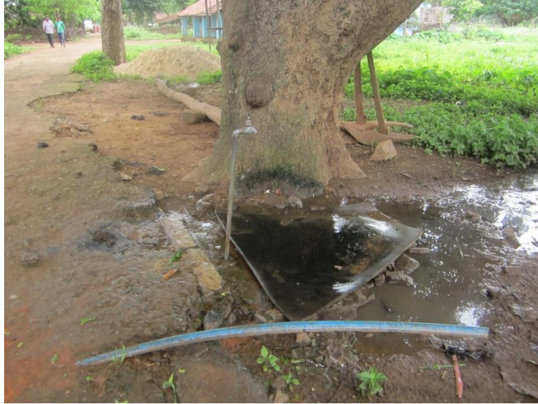
Figure 7: Poor Quality Government Installed Public Stand Post Regularly Clogs Water in the Surrounding Area
