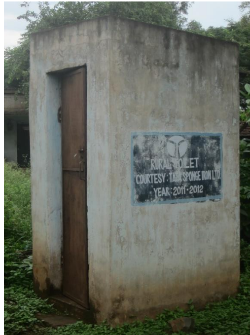
Figure 11: Tata CSR group constructed some toilets in the region. All of these toilets lack water connections required for flushing.
