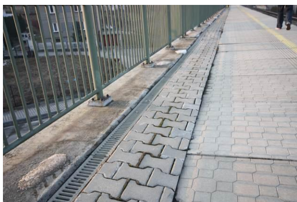
Fig. 6 View in the longitudinal axis of the platform with visible deformations. Photo A. Poláček.
