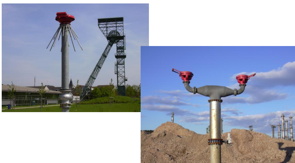
Fig. 4 Degassing plant at abandoned shafts in Germany [7]
