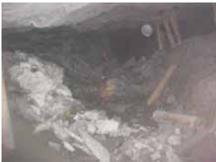
Fig. 14 Larger event magnitude ejects rock even into the gully (note dislodged support units as a result of thrown rocks)
