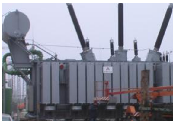
Fig.1 The autotransformer 400/121/34 kV
