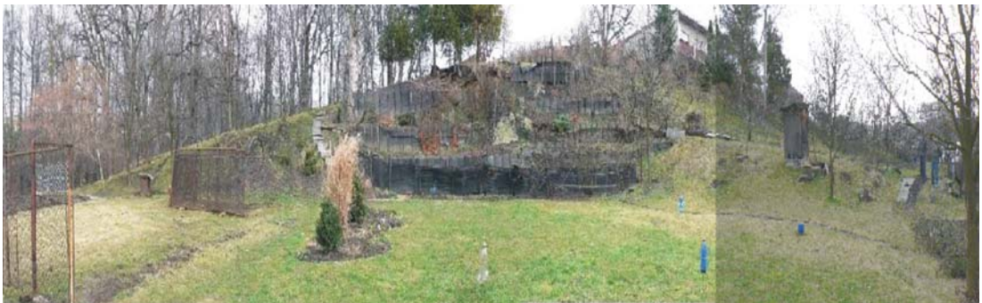
Fig. 4: Tear edge of the slide
