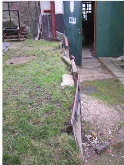
Fig. 8: Sliding and displacement of the top soil near the workshop
