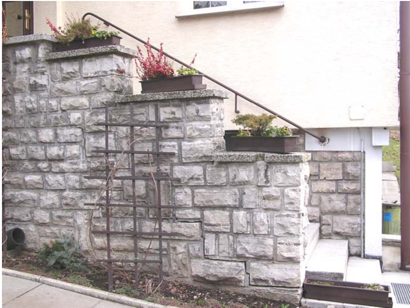
Fig. 5: Damage to the construction of the house
