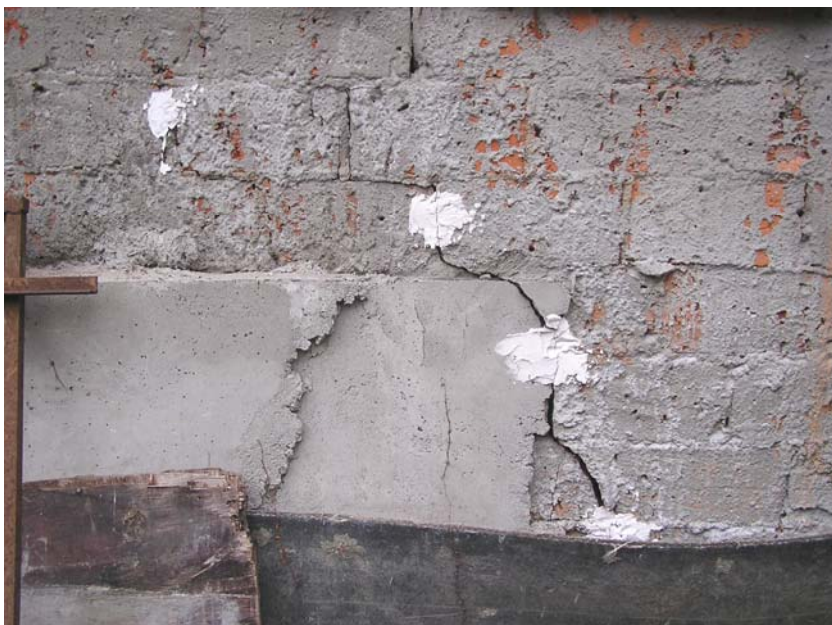
Fig. 6: Damage to the construction of the workshop
