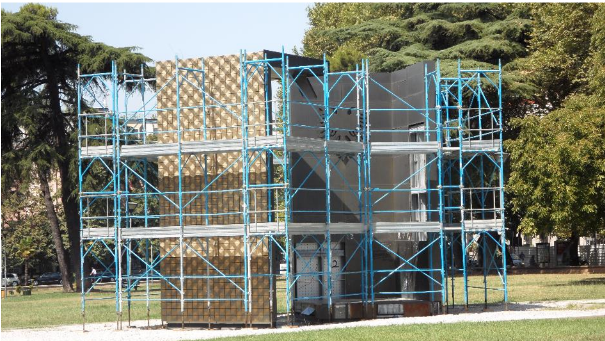
Figure 4. The scaffolding surrounding the Tirana Independence Monument, photographed in summer 2015. Photo by the author.
