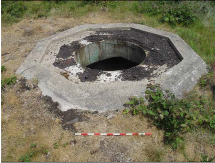
Plate 5.23. One of the Tobruk pits located on Longy Common (author's own photograph)
