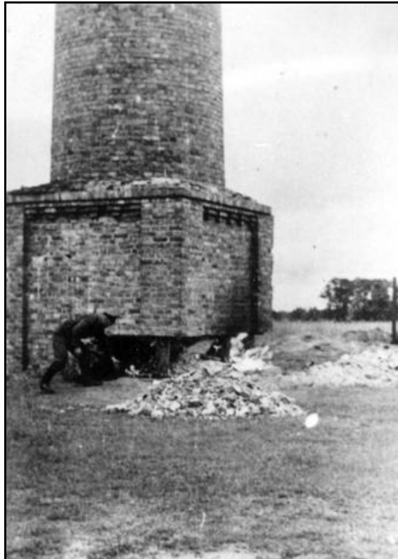
Plate 4.25. A tower in Małkinia being demolished to allow the bricks to be used in the construction of the gas chambers at Treblinka II (after YV 1448b)
