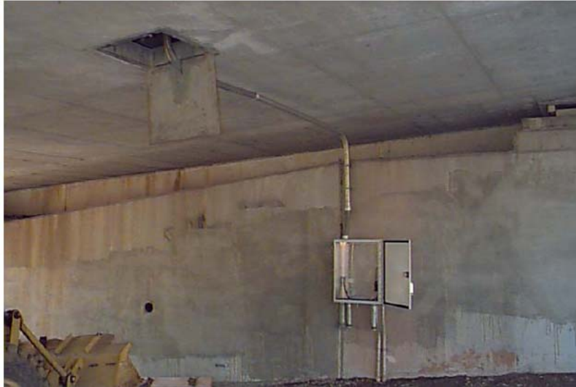
Fig. 3. Example of how bridge monitoring elements are mounted.
